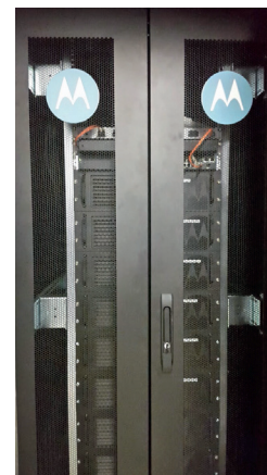
MOTOTRBO DR 3000 repeaters in indoor rack closet
