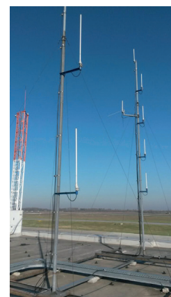
Roof top antenna system
